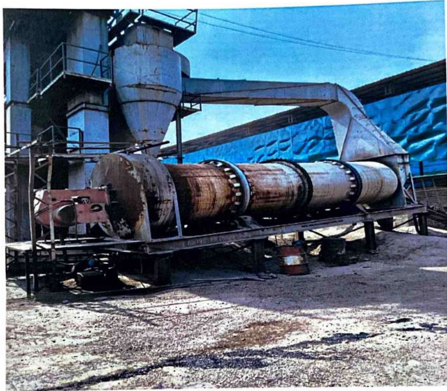
Photo: Hot mix Plant
